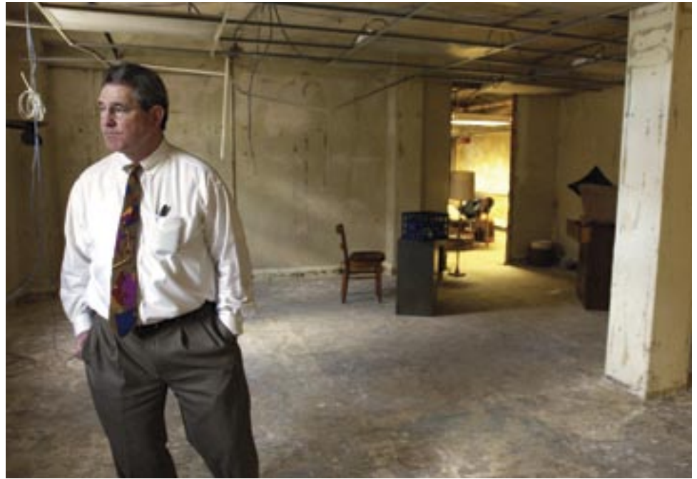
Pierre DeGruy, Jesuit High's development director, is part of the crew aiming to complete major repairs by mid August, the start of next school year.
